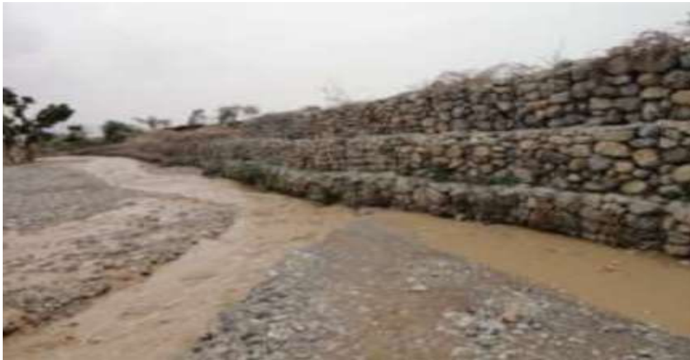
Figure 6. Improved Gabion basket for river diversion (Solomon and Abebe, 2012).
